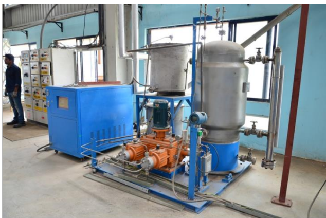
Middle tank and temperature control vessel
